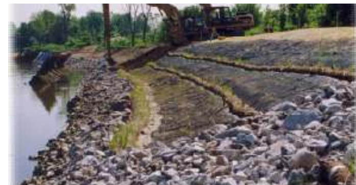
Looking Upstream after First Flood May 2003
