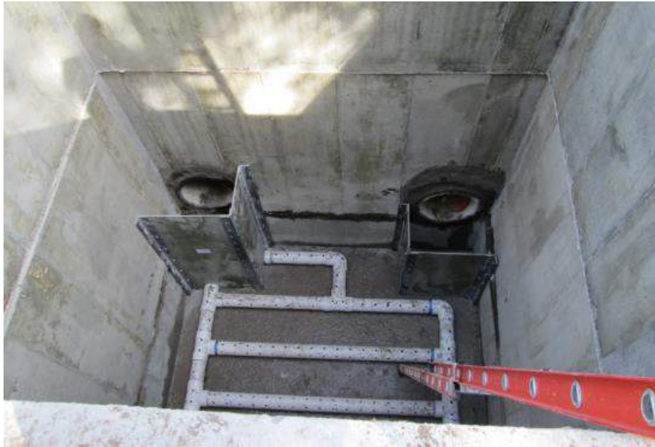
Figure 6-5 Up-flow Off-Line Sorption Filter before Media Placement
