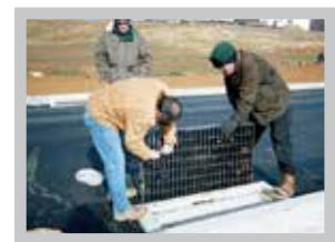
Floc Logs are placed within the drainage system to treat runoff.
