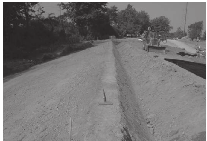
Proper excavation, grading and compaction is critical to the performance of the ACB system.
