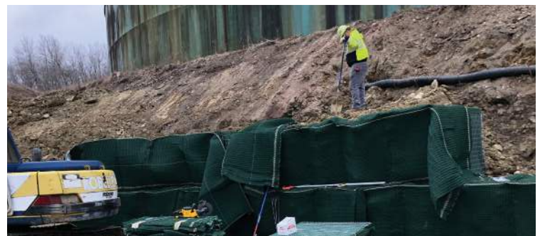
Second layer of Scourlok being covered with soil following being filled (1 cell deep).
