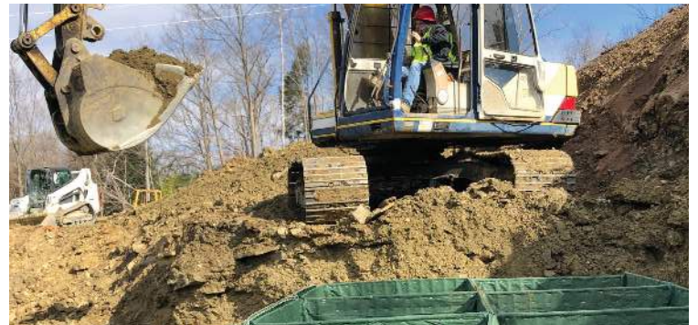
Limited space on site for installation.
