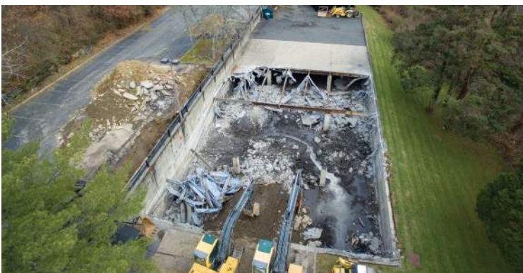
Prior to installation
