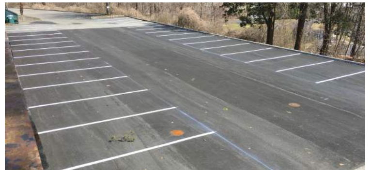
Biaxial geogrid and base gravels are placed before the final asphalt layer.
