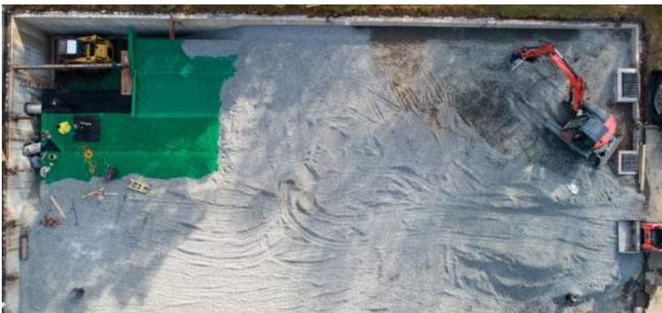
Crushed stone cover layer placed over the tanks and SR-18 microgrid prior to final layers.
