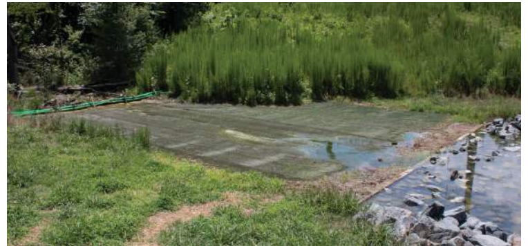
After hurricane—emergency spillway.
