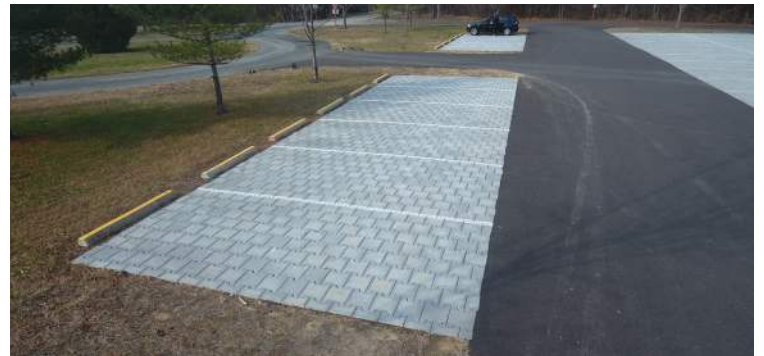
Asphalt drive aisle paired with PowerBLOCK.
